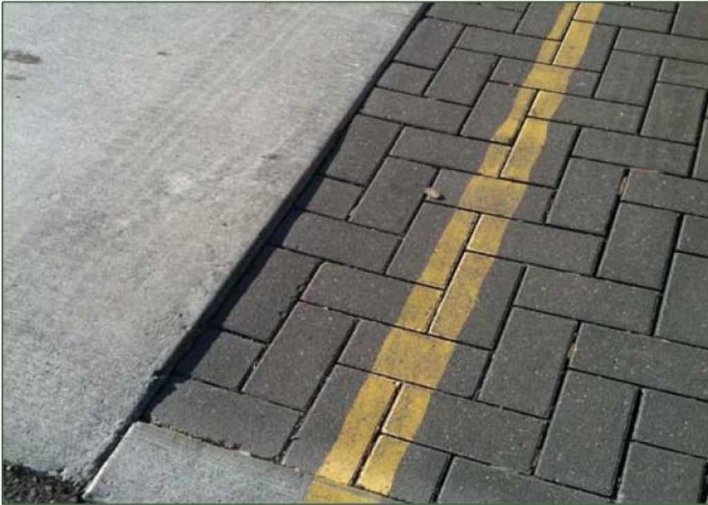
Settlement of Base/Subbase
