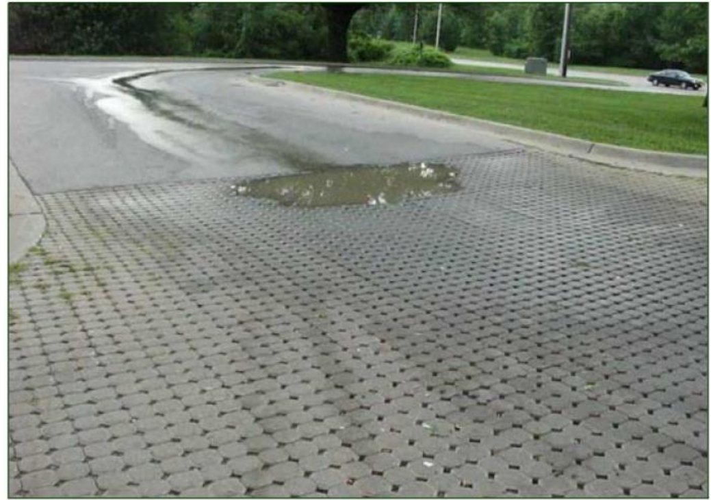
Settlement and Ponding at Transition
