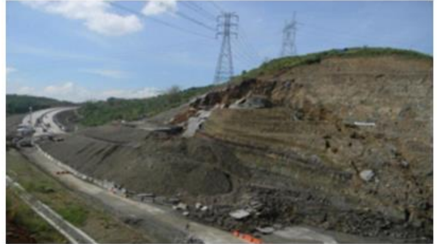
Figure 2 Slope failure at Toll Road Semarang-Bawen, Central Java, Indonesia (Himawan, 2011).
