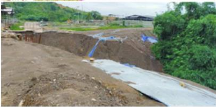
Figure 1 Slope failure on compacted weathered clay shale embankment at Cariu, Jonggol, West Java, Indonesia (Alatas, 2020).
