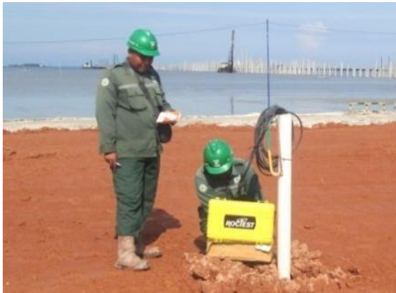
Gambar 69. Monitoring pneumatic piezometer
