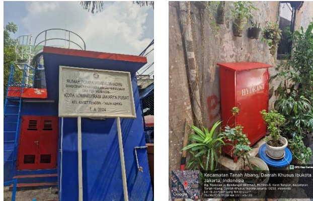
Figure 9. Community-Based Hydrant Houses and Boxes in Karet Tengsin Source: Observation, 2025
