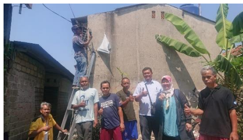
Figure 11 Documentation of the smart cctv system monitoring in rw 19, kampung Lio, Depok
