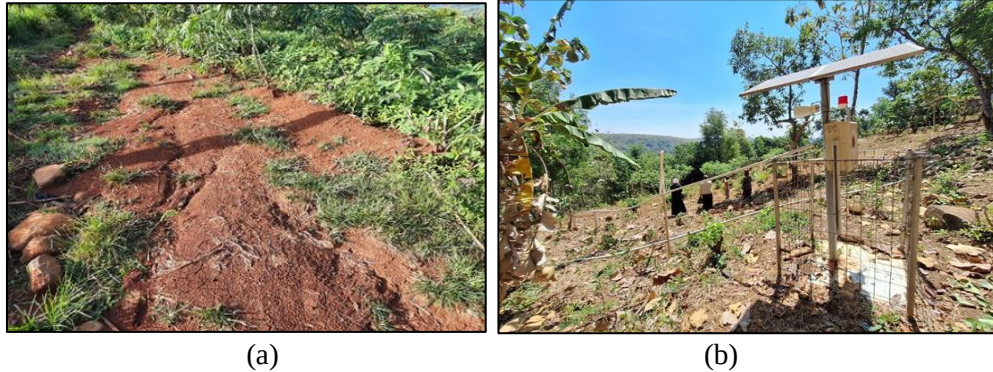
Figure 1 (a) Soil cracks in Sawahan Nganjuk and (b) Cracked soil detection tool in Sawahan, Nganjuk
