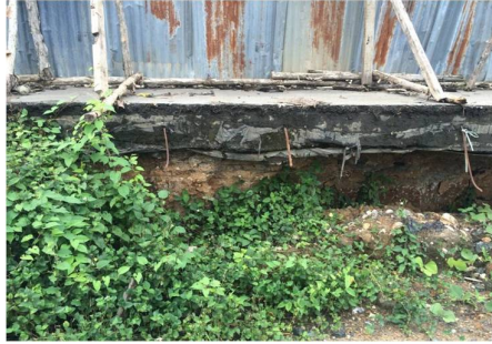
Figure 7. Part Jalan Broken Due Avalanches
