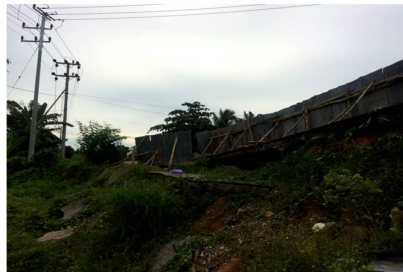
Figure 4. Soil landslide Next to the Canyons
