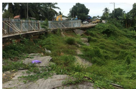
Figure 6. The road Collapsed Due to Avalanche
