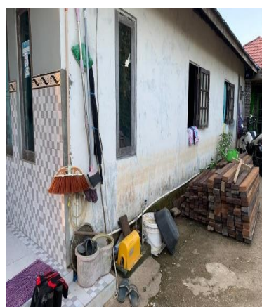
Figure 4. Documentation of Former Flood Heights in Mekar Village
