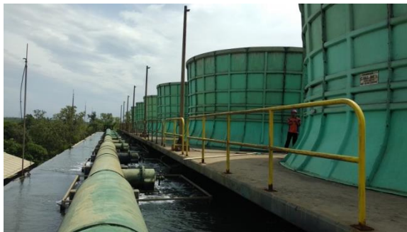
Gambar 1. Cooling Tower Unit 1 & 2 PLTU Asam Asam
