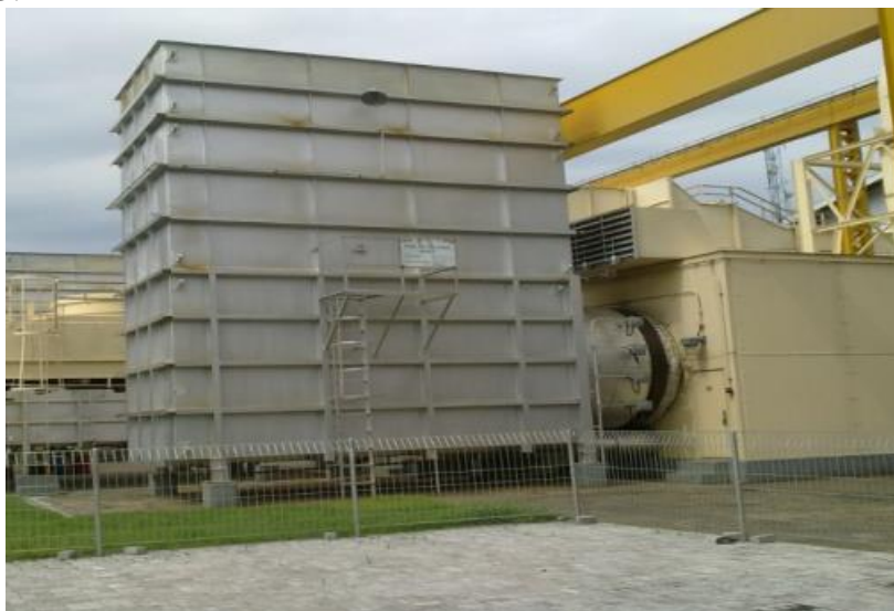
Gambar 3. Air Inlet Section PLTG Unit 4
