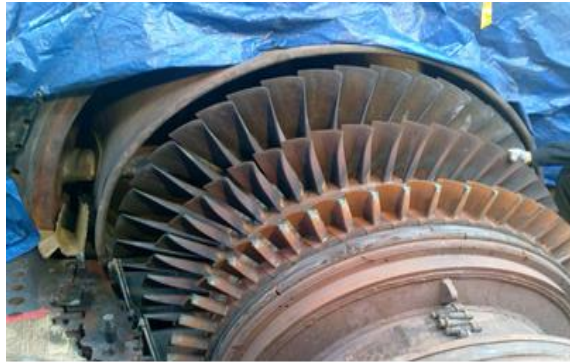
Gambar 6. Turbin Section PLTG Unit 4
