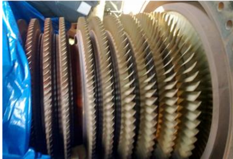
Gambar 4. Compressor Section PLTG Unit 4
